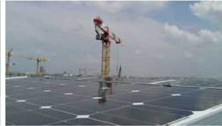
PV panels located in Lyon Confluence on which the "Accusine" solution was tested.
