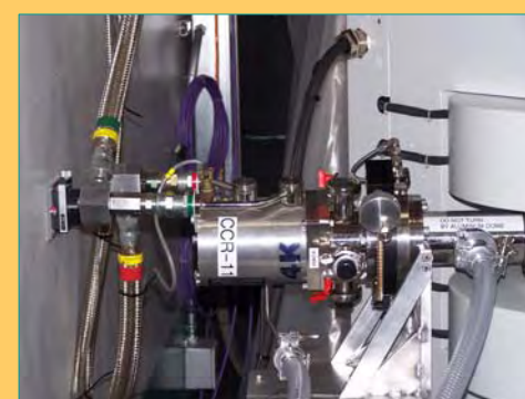
CCR-11 mounted and attached to remote compressor. Even with cable tray removed hoses could not have fit into allotted space.
