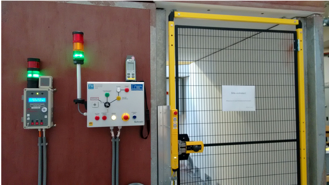
(a) The interlock's control unit and lattice door for access control
